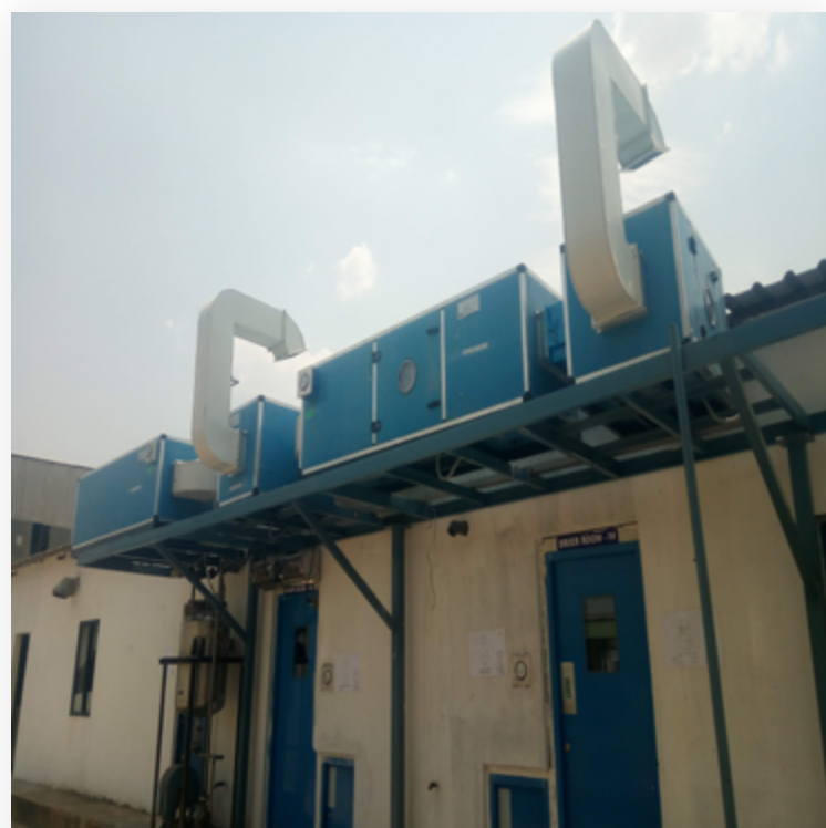
Air Handling Units
