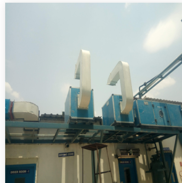
Air Handling Units
