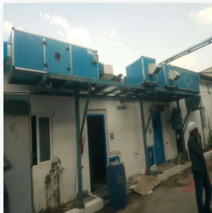
Air Handling Units
